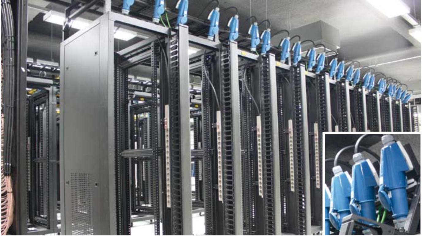
Internet Data Center, Seoul, South Korea
