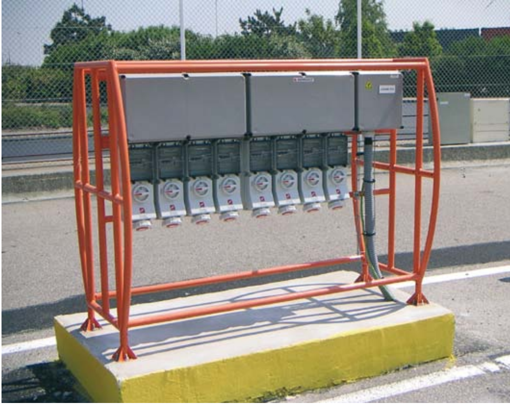
Container Terminal, Le Havre, France
