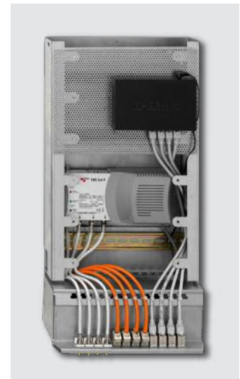
...or with separat Multimedia patch panel
